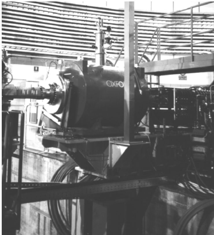
Figure 3 : A Solenoid Compensator Magnet installed in the DAΦNE Hall.
