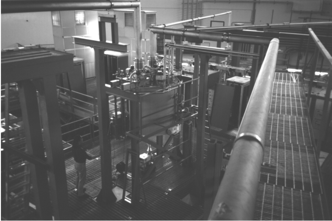
Figure 5 : A view of the Valve Box with the Cryogenic Transfer Lines installed in the center of the DAΦNE Hall.
