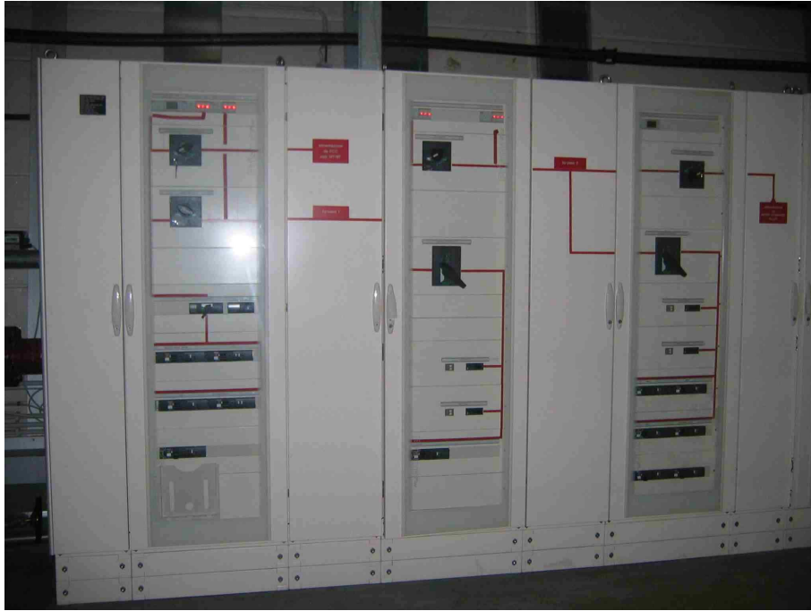
Figure 1: Main cabinet at the entrance of Hall C.
