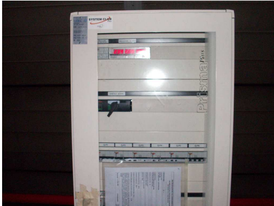
Figure 3: The main power switch.
