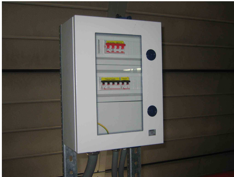
Figure 9: One of the two BMS cabinet located on the top platform.
