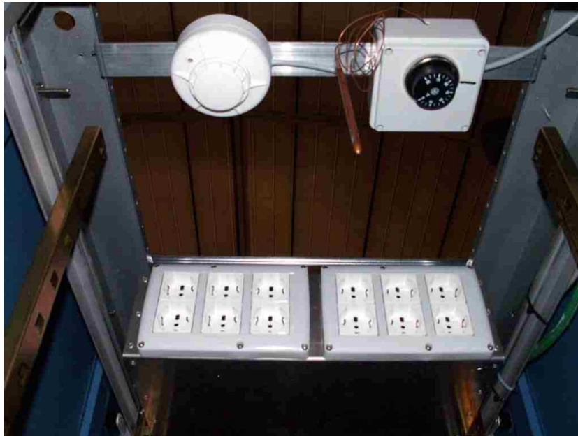
Figure 6: Temperature and smoke sensors. The knob allows the regulation of the overtemperature alarm threshold. The back of the distribution box and the corresponding plugs are also visible.
