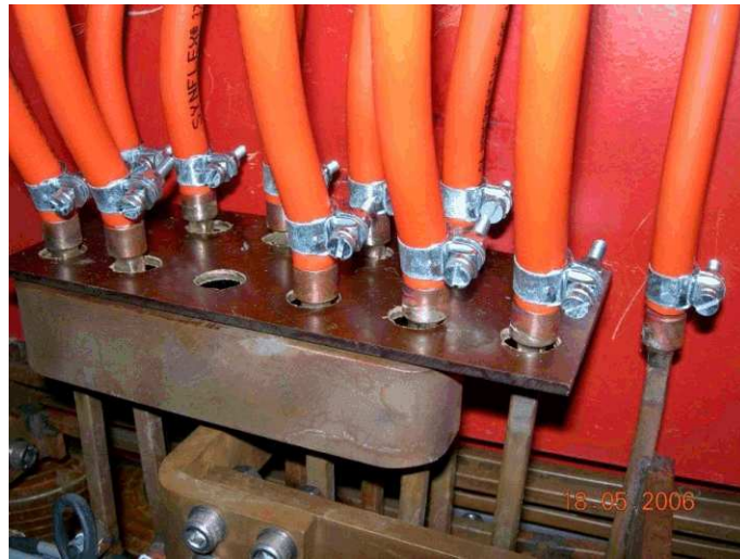
Figure 5: Wiggler cooling system upgrade.
