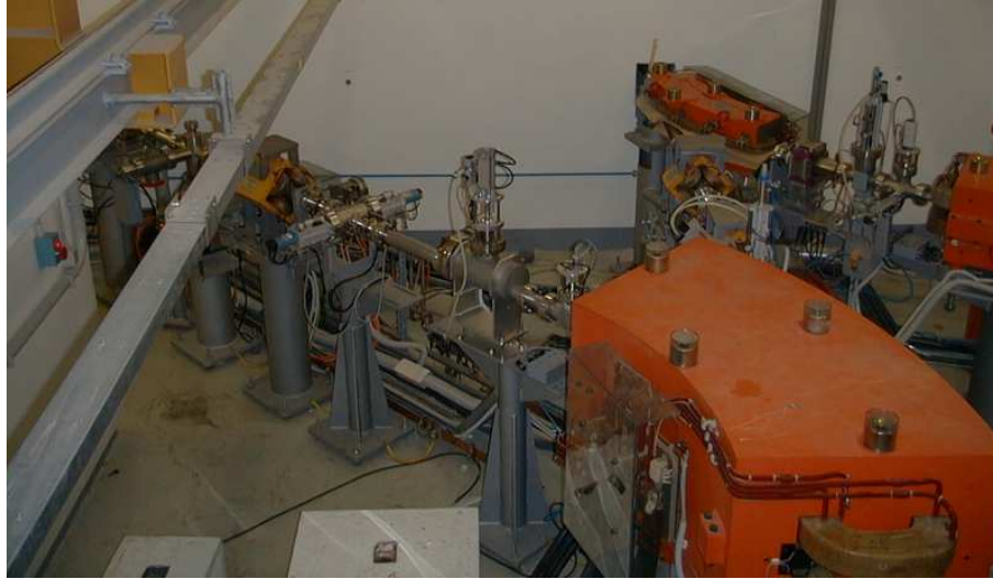
Figure 5: Photograph of the transfer line to the BTF (in the LINAC tunnel). On the left, from the foreground: the bending magnet of the selector (DHSTB01), followed by a “flag” (FL1TB01), the slits (SLTTB01) and a quadrupole (QUATB01); on the right, in the background, the transfer line of the accumulator ring (DHPT02).
