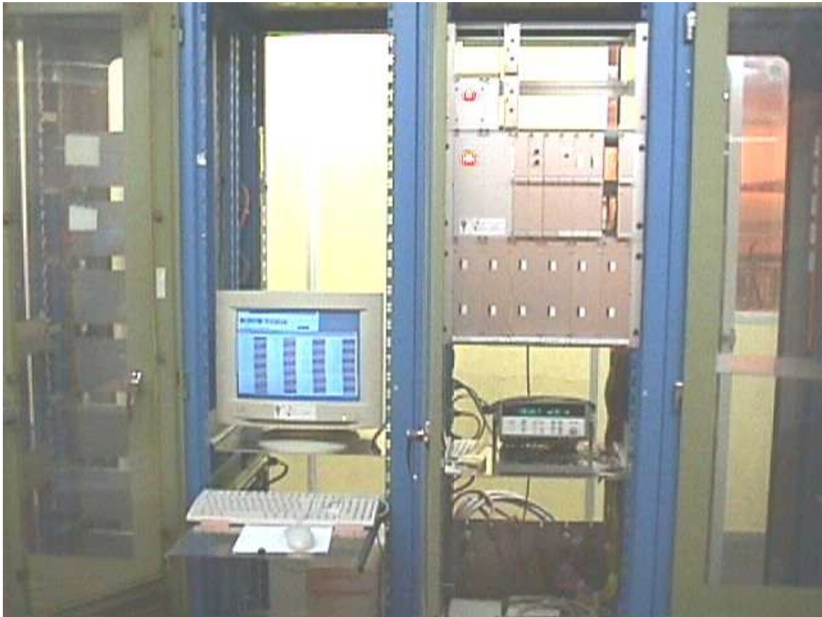
FIG. 10 – The LASA-DAQ system in the CERN control room (Bldg. 180).
