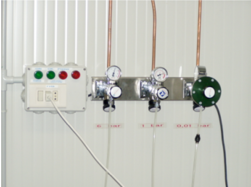
FIG. 6: The gas lines.
