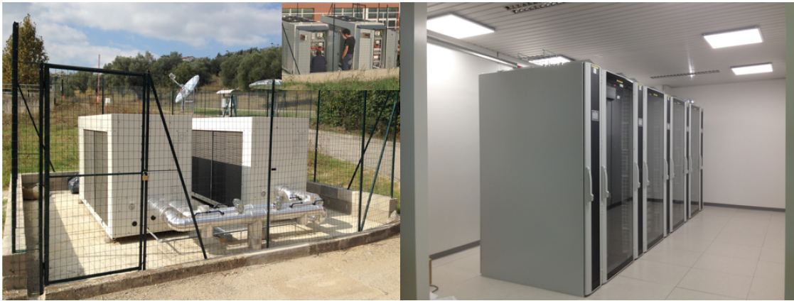
Figure 1: (Left) The two-Chiller system (with integrated free cooling) installed at the ReCaS Cosenza Site. (Right) The white space and the racks (with LCPs) hosting part of the IT equipment.
