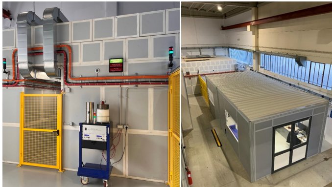
Figure 1: TEX Concrete bunker entrance (left) and top view of the control room and the bunker (right).
