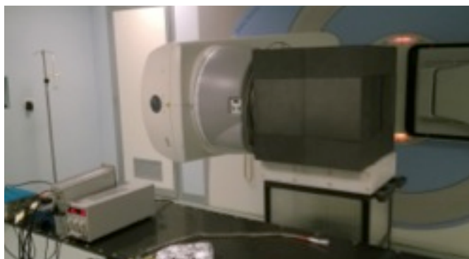
Figure 1: Linac and photo converter / moderator installed at S. Luigi Orbassano Hospital
