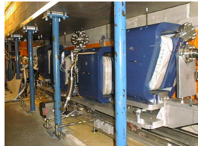
ATF bunch compressor installed in tunnel.
