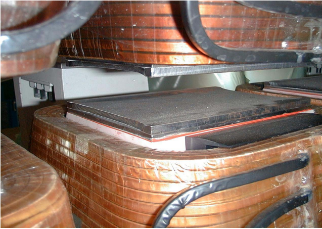
Additional plates glued on wiggler poles
