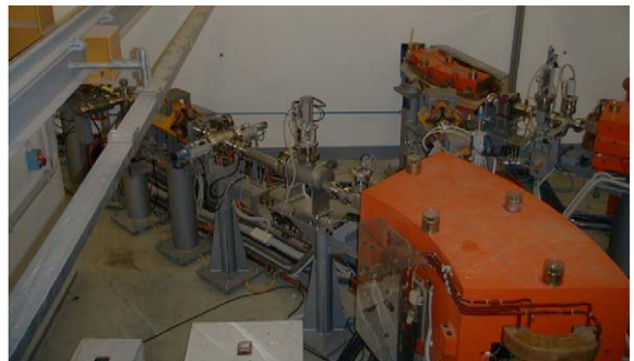
Fig. 4. The BTF transferline inside the LINAC tunnel. On the right, from the foreground: the bending magnet of the energy selector ( Dipole 1), followed by the small vertical tower of a fluorescent screen, by the two horizontal parts of the Collimator 1 and by a quadrupole magnet. On the right, in the background, the transferline from the Accumulator to the Main Rings.
